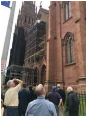
Local architects view ongoing restoration efforts at the Cathedral, including current work on the Rose Window.
